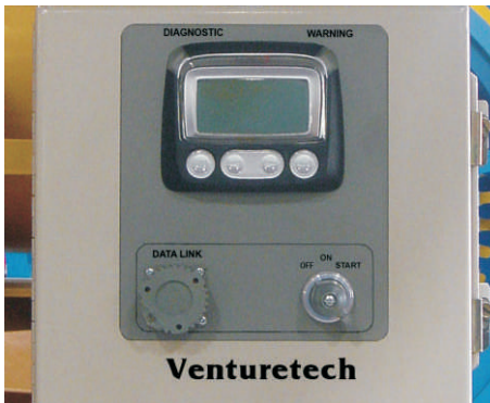
Engine control panel
